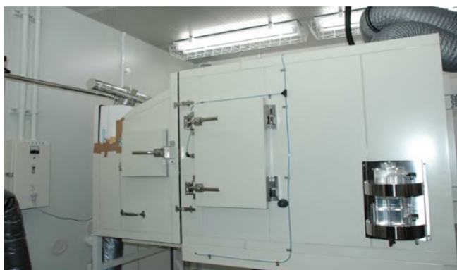
図③.2.1-4 Wind receiving chamber in the indoor unit test room
