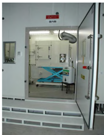
図③.2.1-3 Indoor unit test room
