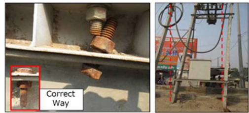
Figure 19: Defective bolt (left), tilted pole (right)
