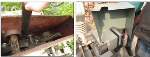
Figure 18: The Gearbox with Water Leakage (left) and Waterproof Cover (right)
