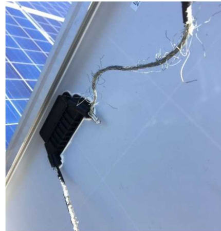
Figure 12 Wire damage due to small animals
