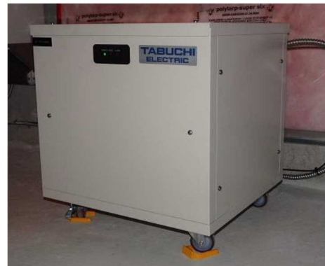
Figure 8 Battery storage unit
