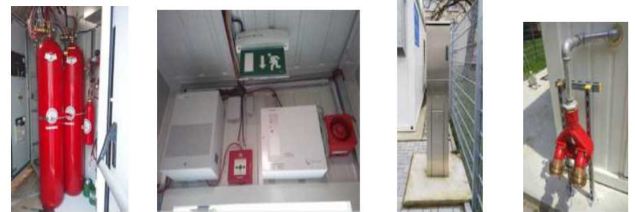
Figure 5 Installation of fire extinguishing gas cylinders, communication equipment to fire stations, fire information control systems (FIBS), and water injection ports
