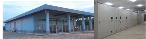
Figure 4 Facilities in the industrial park where HQPS was installed (outer appearance and inside)
