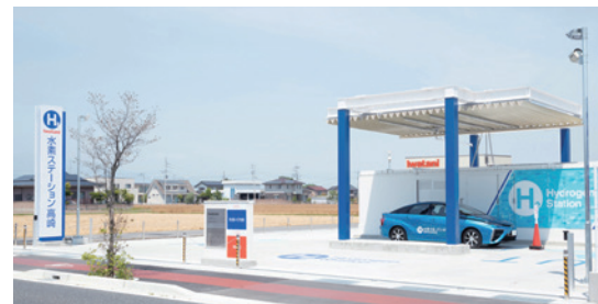
At hydrogen stations, fuel cell-powered cars and buses are refueled. Source: Iwatani Corporation
