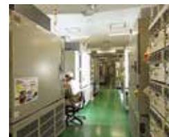
Charge-discharge test equipment occupying most of the room
