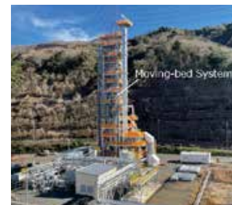
CO 2 solid absorber plant (Courtesy of Kawasaki Heavy Industries, Ltd.)
