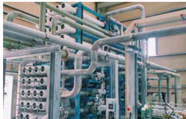
Part of energy-saving seawater desalination system
