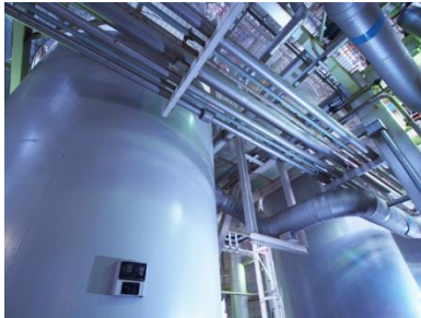
Gas cleanup facility
