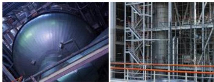
View from the bottom of gasifier (left), side view of gasifier (filled with COS catalyst) (right)
