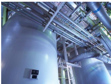
Gas cleanup facility
