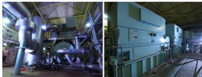
Piping to transport air to gasifier (left), Air-booster compressor (right)
