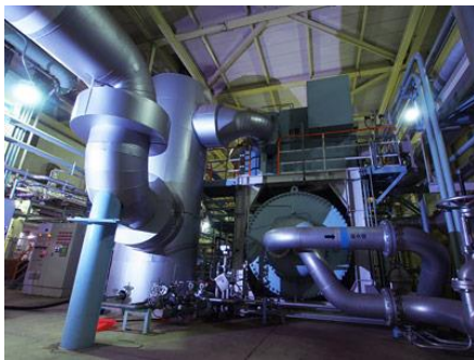
Piping to transport air to gasifier
