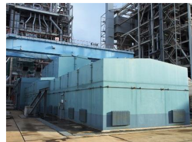
High-efficiency gas turbine combined cycle
