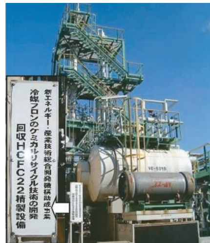
Figure 3 Coolant Purification Facility
