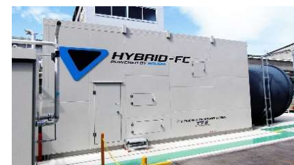
Fuel cell generator
