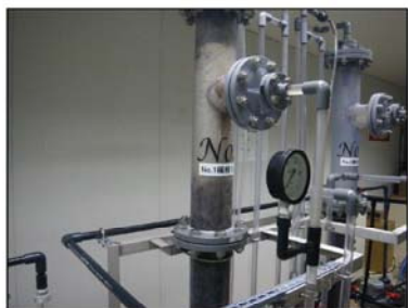
No.1空気逆洗状況
