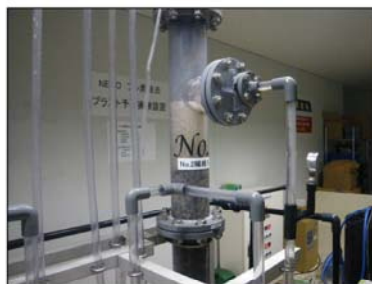
No.2空気逆洗状況
