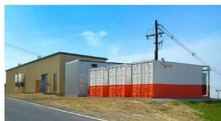
3MWプラント@米国PA州Lyon Station (East Penn社 鉛蓄電池: Ultra Battery)
